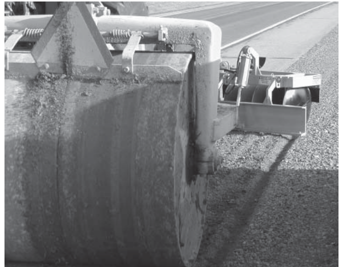
A roller attached by a bar on the back of the same mowing tractor shown above, compresses the recovered stone in place, restoring the berm in one operation. A second vehicle follows behind to provide traffic control.
