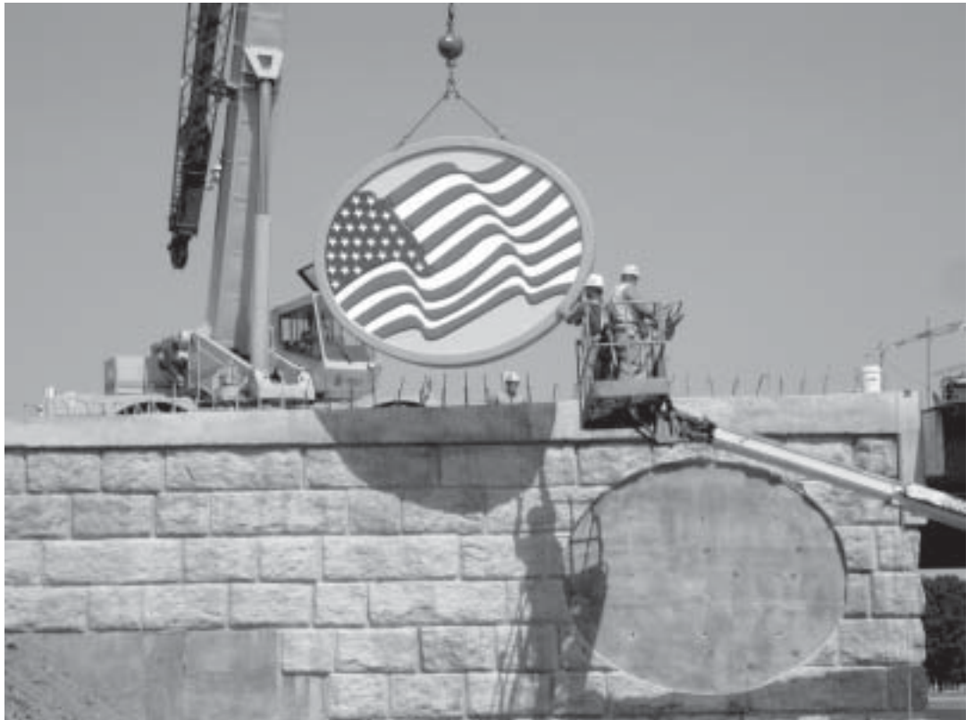
This 9,000-pound medallion, reflecting Findlay's Flag City U.S.A. theme, is one of four that was attached to the State Route 12 bridge over Interstate 75 as part of ODOT's design aesthetic initiative to improve the appearance of the state's highways.
