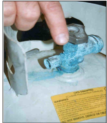
Blue valve means danger!
