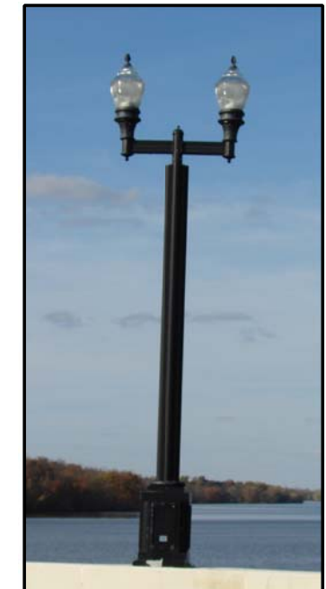
HOME ROAD BRIDGE LIGHTING
