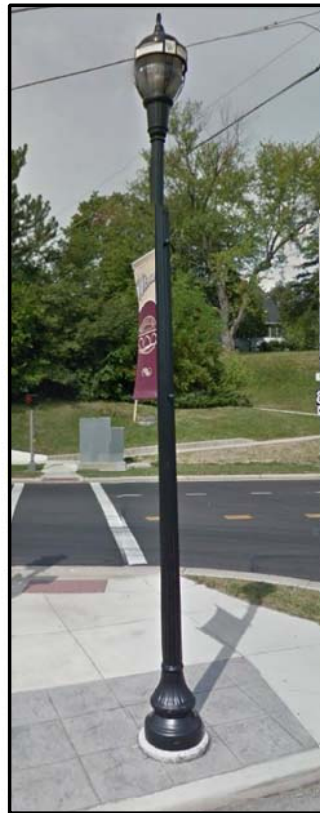
EXISTING WATERVILLE LIGHTING
