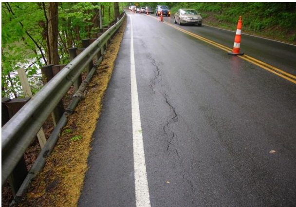
Distress on the SR 315 pavement due to slope instability
