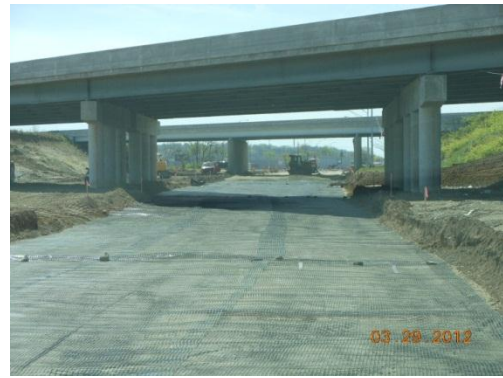
Looking west along Central Ave. under I-75 at the geotextile fabric placed over the subgrade for the new pavement
