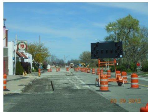
Beginning the pavement removal on Dixie Dr. just east of Alex Bell Rd.
