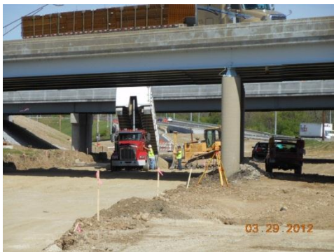
Placing aggregate base for the new pavement on Central Ave. under I-75
