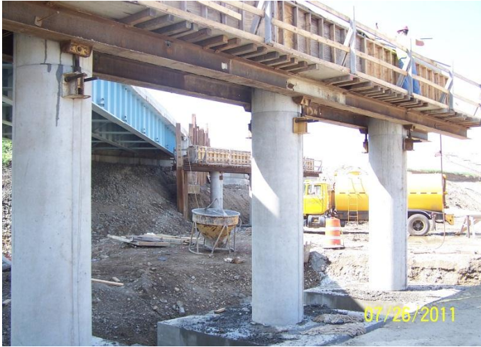
Construction of the new piers on the I-75 northbound bridge over Central Ave.
