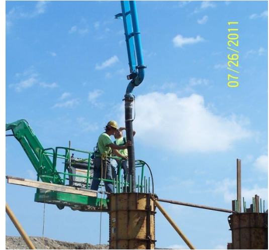
Pouring concrete for the new piers on the I-75 northbound bridge over Central Ave.
