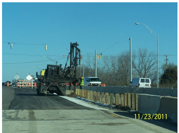
Installing new guardrail posts along Central Ave. just east of the Hole's Creek bridge
