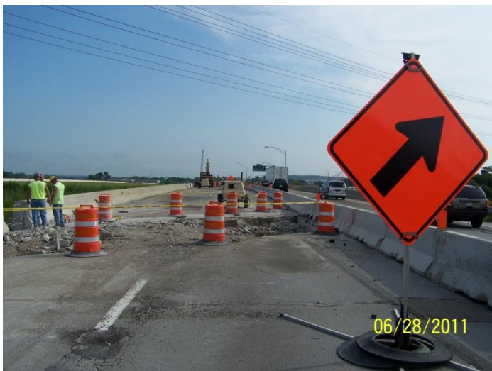
Work on the northbound I-75 bridge over E. Dixie Dr. and the railroad
