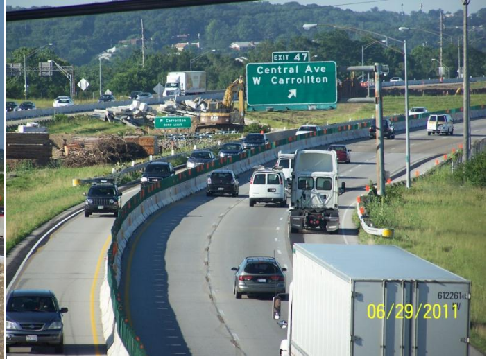
I-75 with southbound lanes on the right and the single northbound lane on the left
