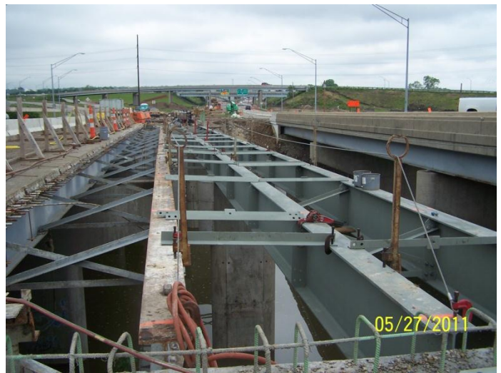
The portion of the Dixie Dr. bridge over Hole's Creek that is being widened, looking west
