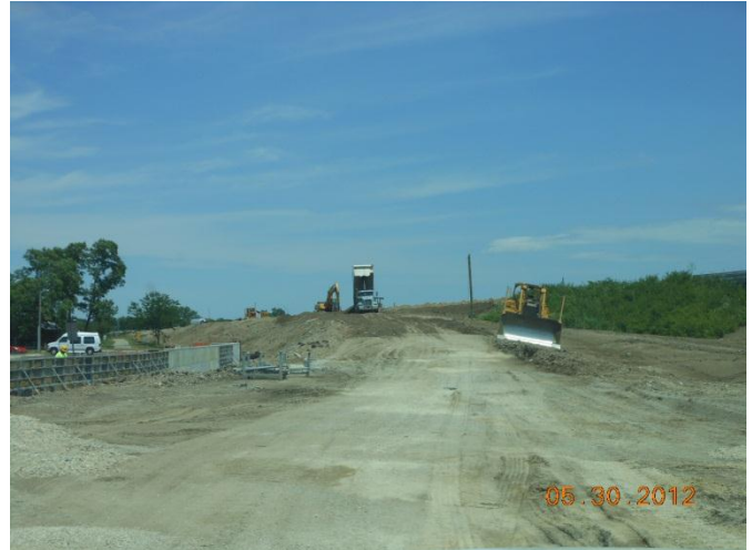
The beginning of the new ramp from southbound I-75 to Central Ave.
