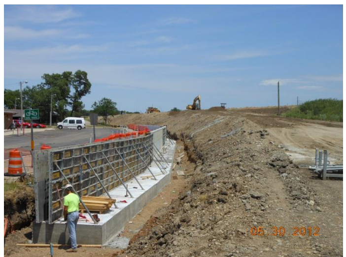
Construction of the new retaining wall along the southbound I-75 exit ramp
