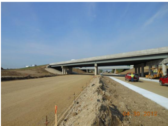
Looking west along the new Central Ave. and Dixie Dr. where they will go under I-75
