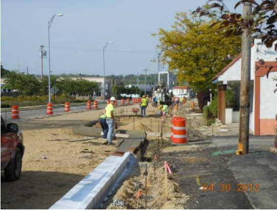
Placing new curb along Dixie Dr. just east of Alex Bell Rd.
