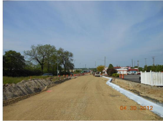
Looking west along the new alignment of Dixie Dr., just west of Marina Dr. , with new curb on the right
