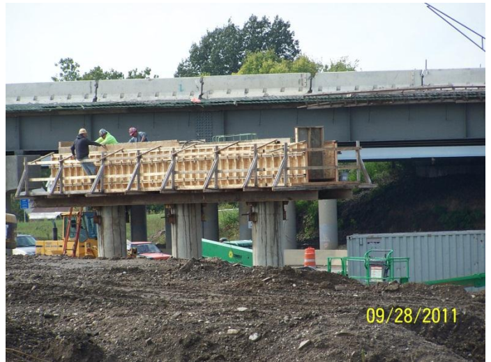
Pouring concrete for the new pier cap for the northbound I-75 bridge over Central Ave.
