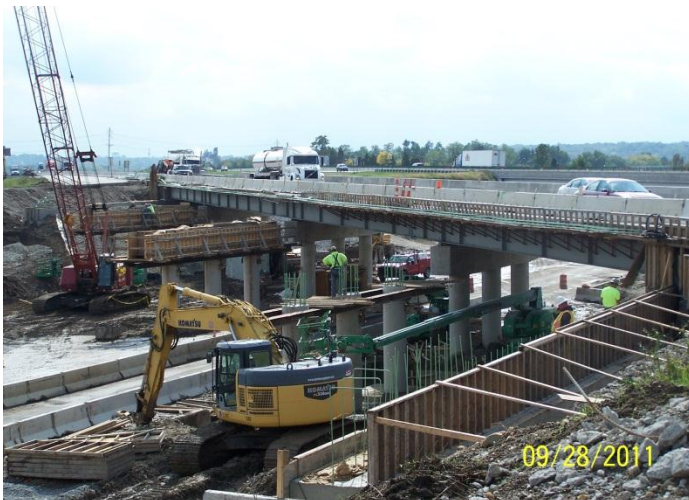
Construction of the exterior half of the I-75 northbound bridge over Central Ave.
