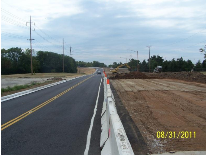
Dryden Rd. looking north with the new pavement and curb on the left and the new roadway going in on the right
