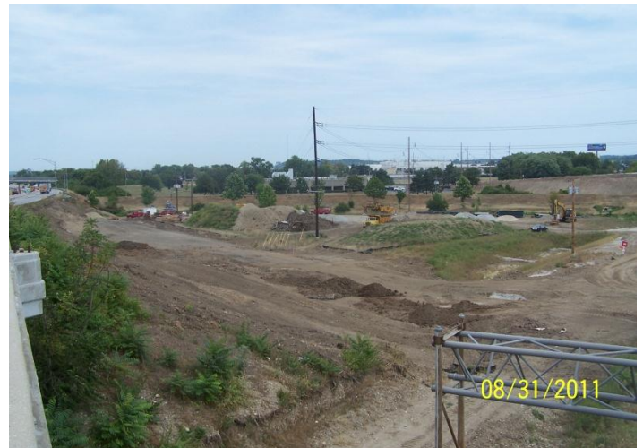
The beginning of work on the new ramp from Dixie Dr. to northbound I-75
