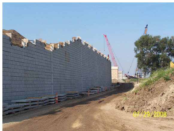
Construction of the mechanically stabilized earth (MSE) wall which will be connected to the new river bridge.
