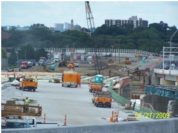
Construction on the bridge over the Great Miami River that will carry traffic on I-75 north and southbound
