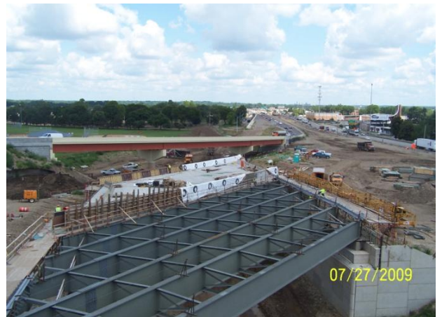
Bridge that will carry traffic from I-75 north and southbound over the exit to State Route 4 north and Webster St.
