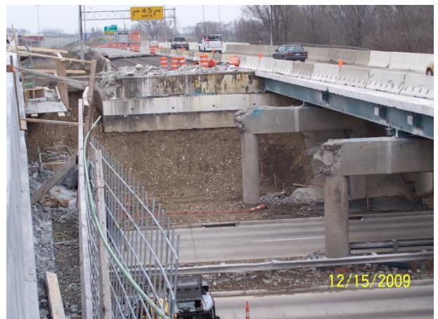
Looking at the new bridge deck over Main St. that is waiting to be poured.
