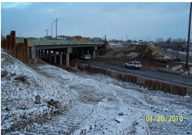
Looking at new construction for a bridge to carry I-75 northbound traffic over Keowee St.
