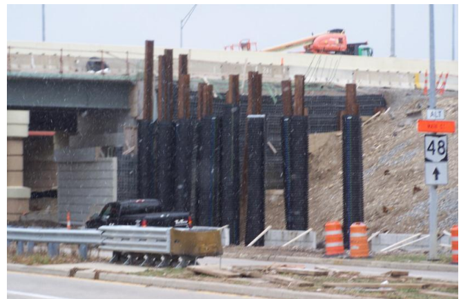
The forward abutment piling at the bridge along Riverside Drive that will carry traffic from I-75 northbound to SR 4 northbound
