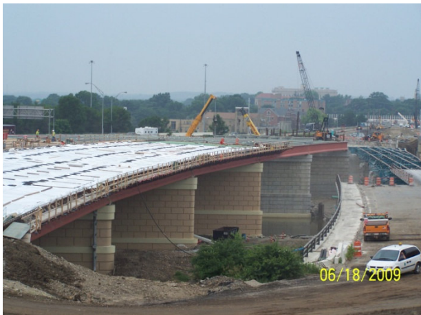
This photo shows the new I-75 bridge over the Great Miami River that will carry north & southbound traffic.
