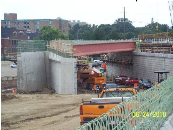
Looking at the new bridge that will carry I-75 NB traffic to SR 4 NB.
