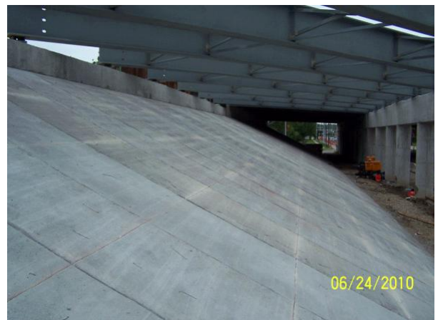
Looking at the concrete slope protection for the new I-75 bridge over Keowee Street.
