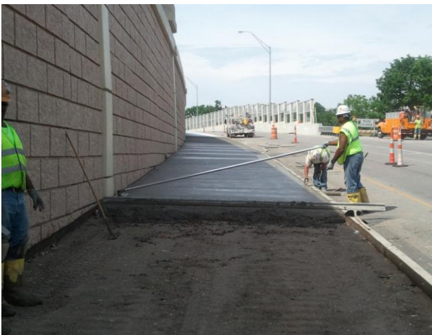
Kokosing continues to pour concrete for the new pavement on NB Main St. at I-75
