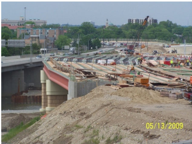
Decking the mainline bridge over the Great Miami River which will carry northbound and southbound traffic.
