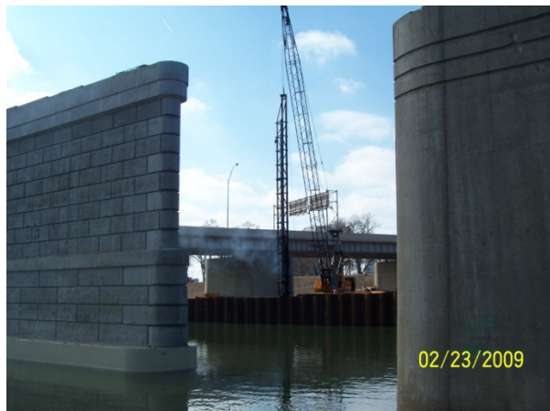
Piling being driven for the I-75 bridge over the Great Miami River
