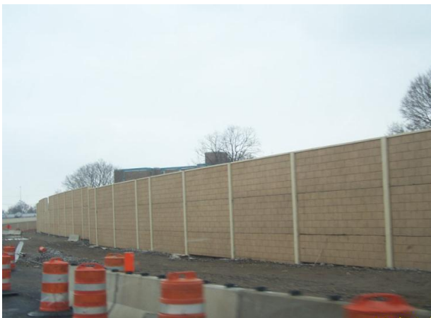
The newly constructed noise wall on the exit ramp from I-75 northbound to Main Street
