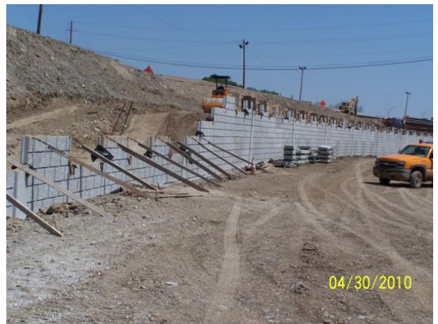
Looking at construction of MSE Wall 2 along the exit ramp from I-75 NB to Main St.
