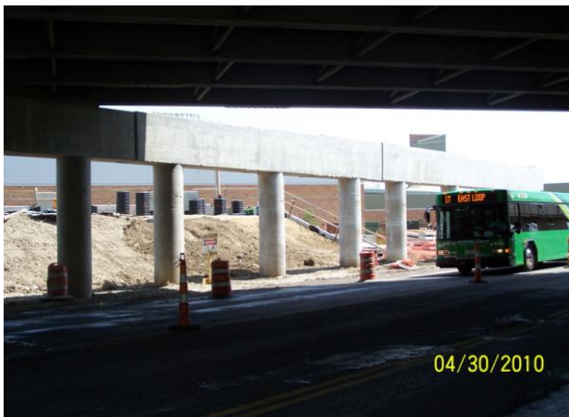
Looking at new bridge piers that will carry I-75 NB over Keowee St.
