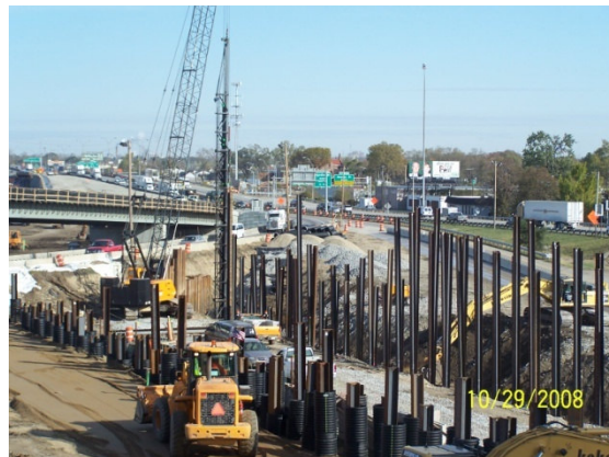
Piling in place for the new ramp from I-75 south to SR 4 north
