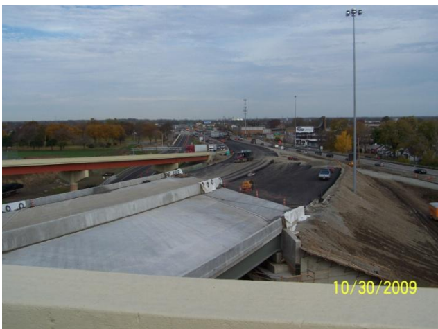
Looking at the bridge which will carry I-75 north and southbound traffic over the State Route 4 northbound off ramp.
