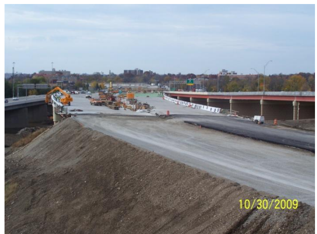
Looking at the bridge over the Great Miami River that will carry both north and southbound I-75 traffic.
