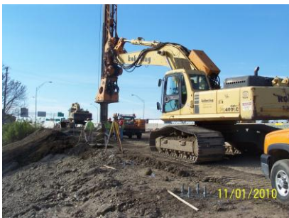
Looking at noise wall foundations being drilled along the ramp from I-75 NB to Main St.
