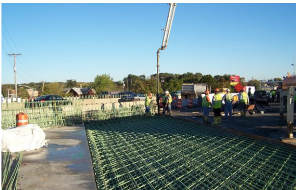
Looking at I-75 NB over Keowee St. as crews pour concrete for approach slabs.
