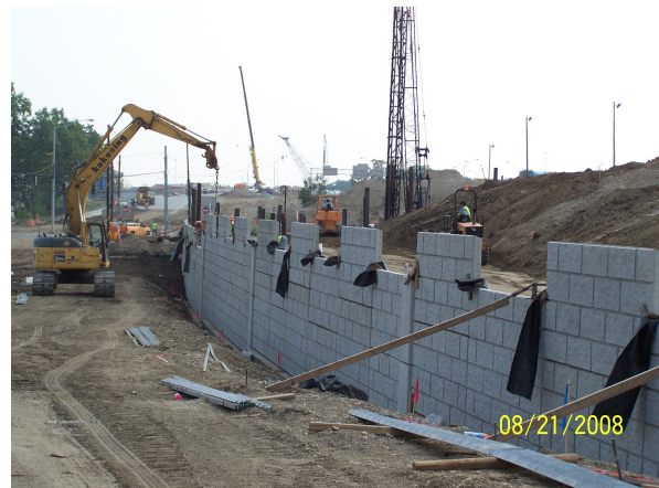
Construction of mechanically stabilized earth wall along the future mainline of I-75
