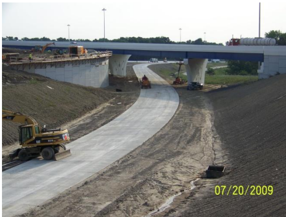
Looking northeast at the future ramp of I-75 SB to I-70 EB going under the flyover ramp.
