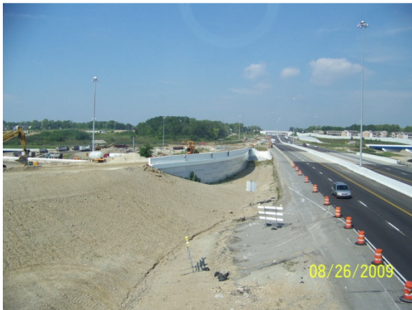
Looking west at the future ramp of I-70 EB to I-75 NB (top) and part of the closed old ramp (bottom).
