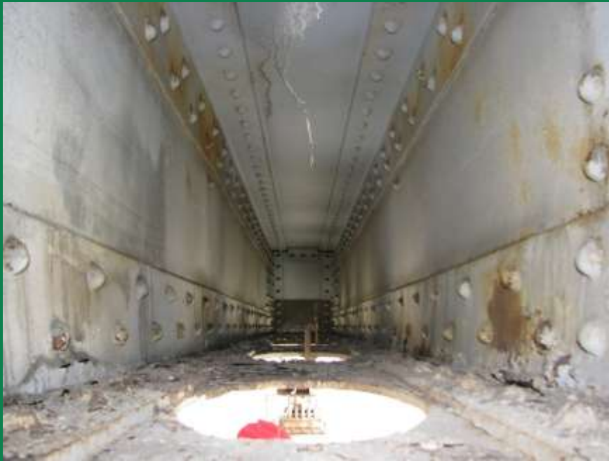
(Above) Inside of affected member (L300-L301S).
