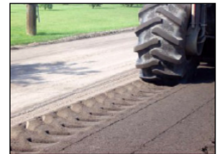
Material before mixing (left) and after mixing (right). Note the fly ash on the left side.
