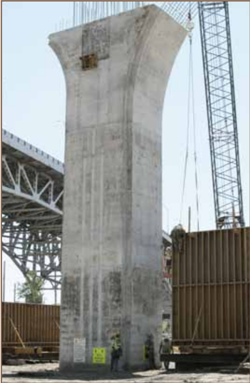
This pier is now ready for the pier cap form to be set on top, bridging between the two legs of the pier.
