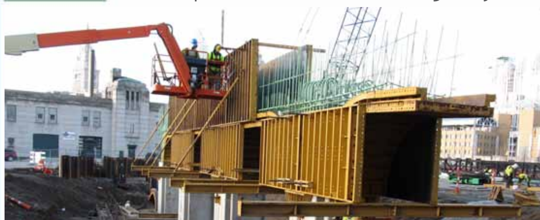
Top: Carpenters, ironworkers and laborers all play a role in preparing this bridge (I-90 west over E 9th St) for pouring the concrete deck. Bottom: Carpenters work to assemble the pier cap forms on Pier 13.
